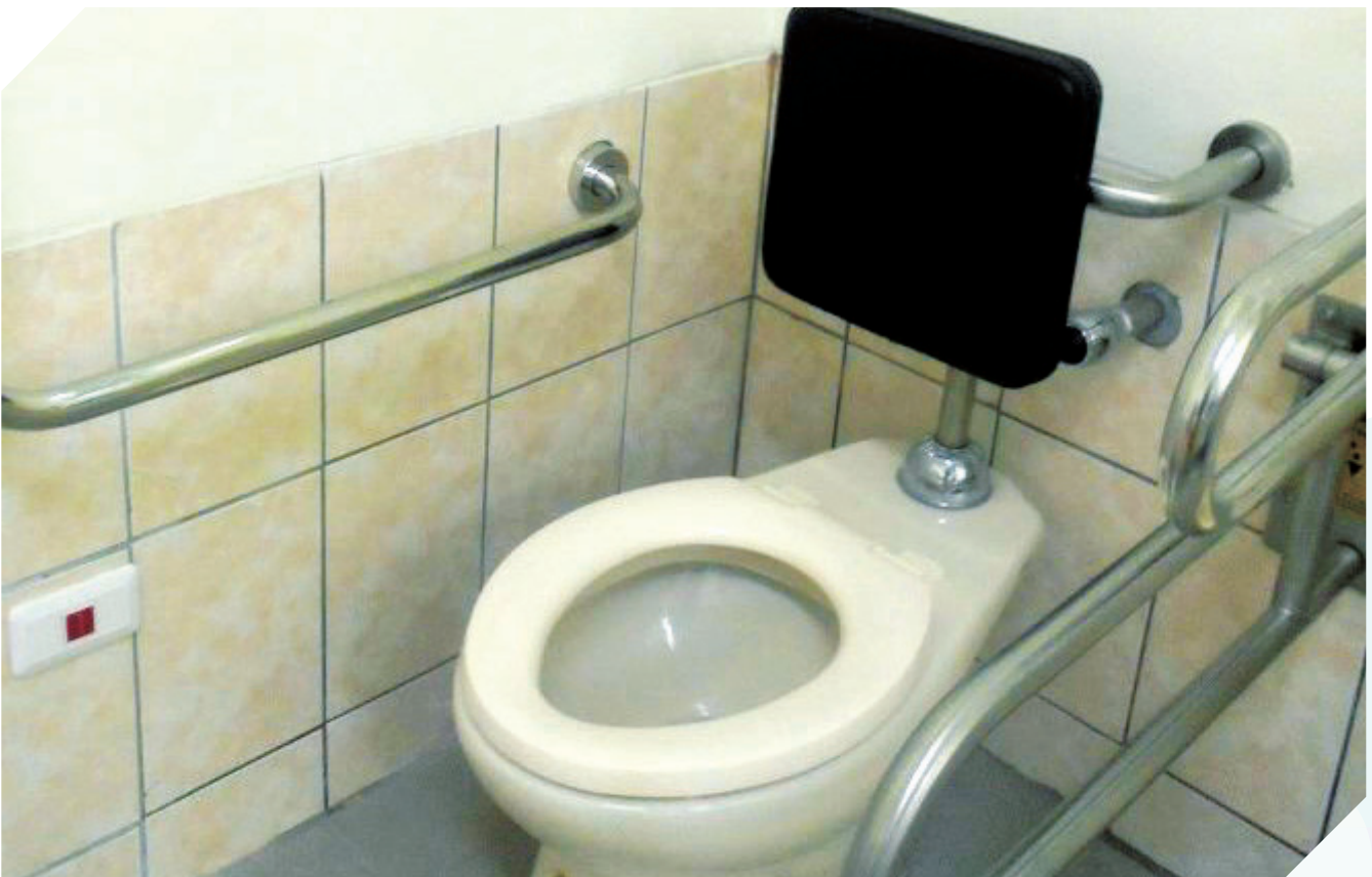
臺南第二監獄舍房建置坐式馬桶及扶手 Tainan Second Prison has installed pedestal toilets and grip handle in the living quarters.
