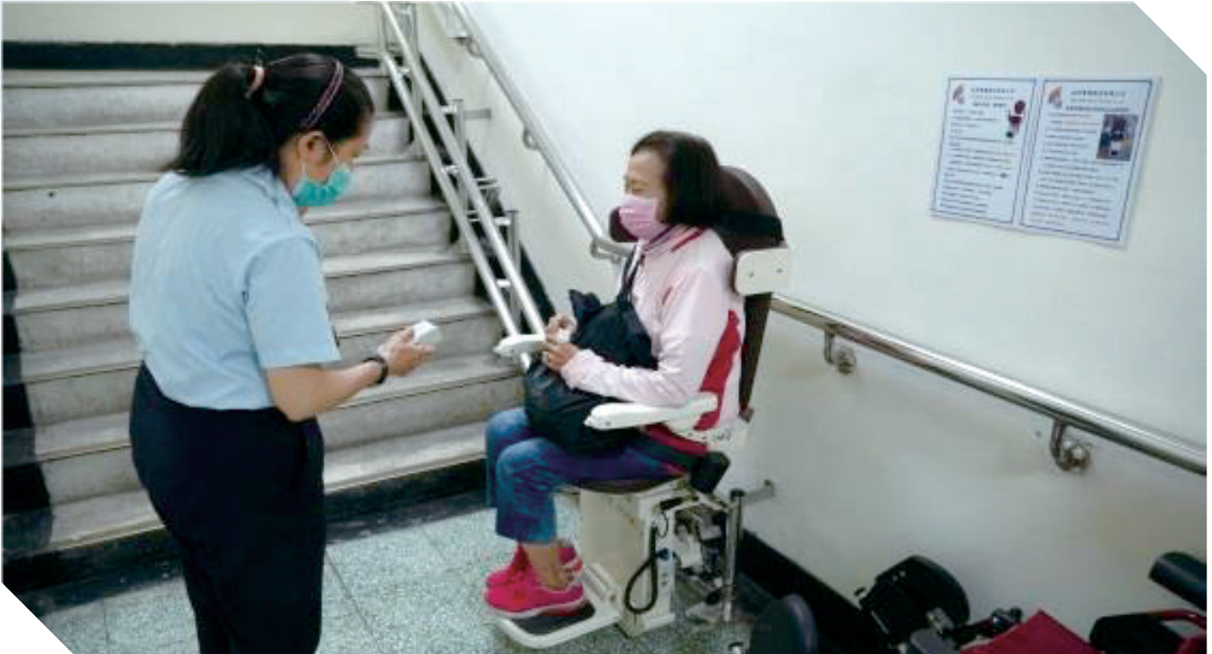
高雄第二監獄建置電動升降梯 Kaohsiung Second Prison has installed an electric lift.
