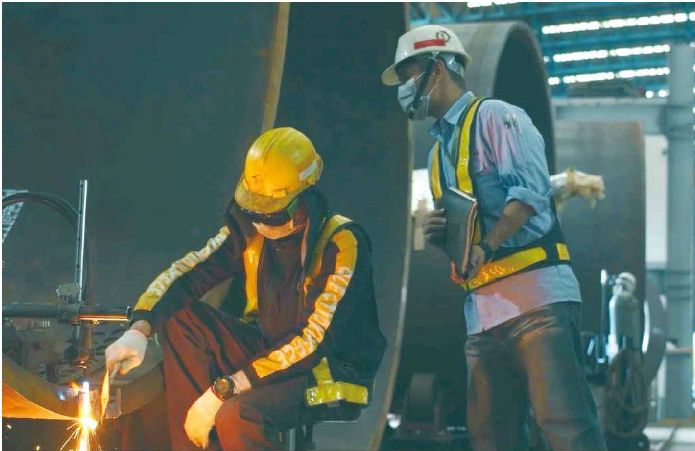
八德外役監獄自主監外作業 - 電銲切割 Out-of-prison work for inmates from Bade Minimum-Security Prison – arc welding/cutting
